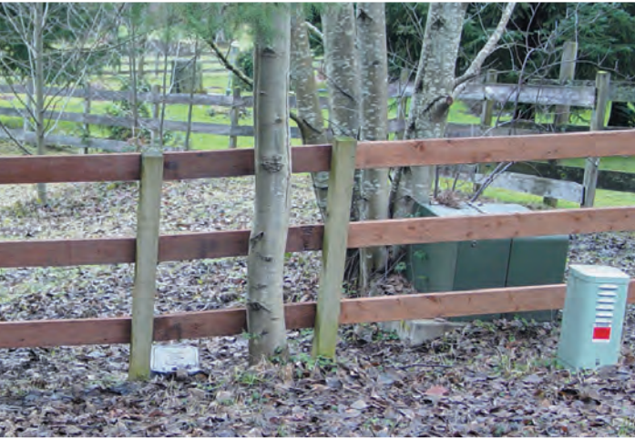
Meter access is obstructed – it's located inside the fence
