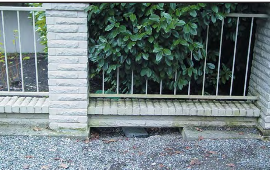
Meter is located underneath the fence
