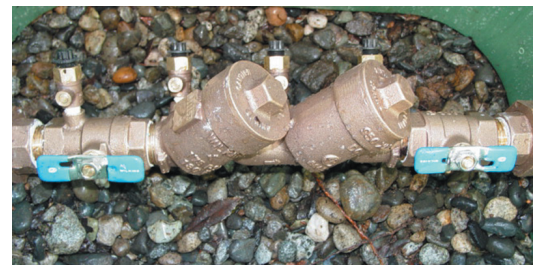
Double Check Valve Assembly used for backflow protection on irrigation systems
